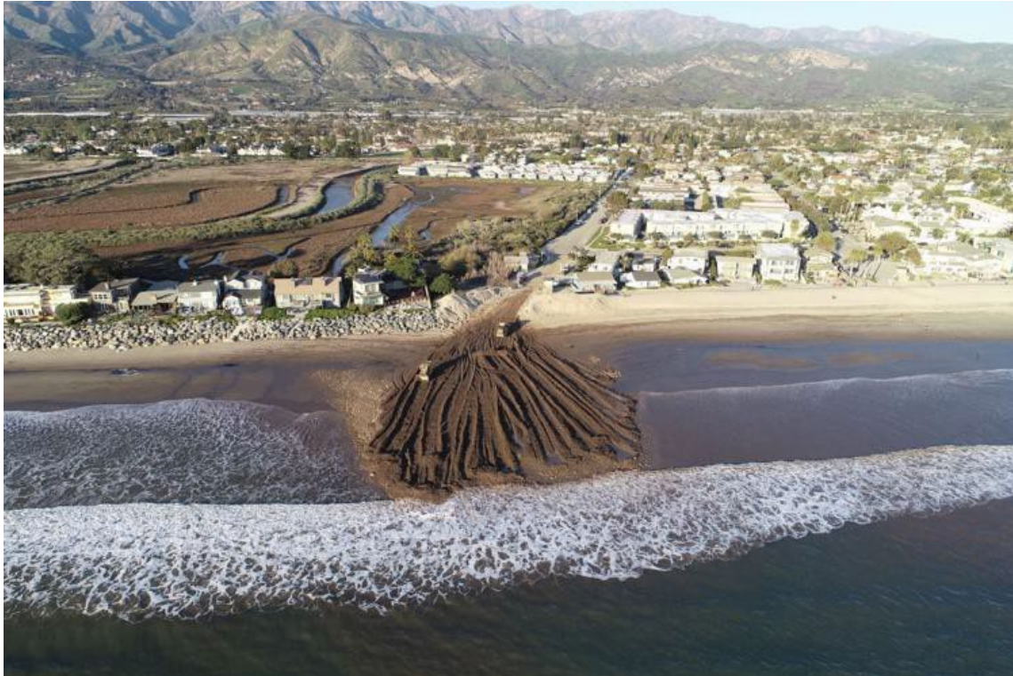
Figure 28. Image of sediment debris flow placement at the end of Ash Avenue in Carpinteria
