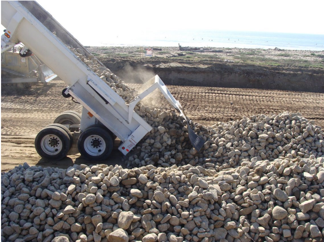
Cobble Placement during construction of Surfer’s Point Living Shoreline Project Phase 1. Photo courtesy of Paul Jenkin
