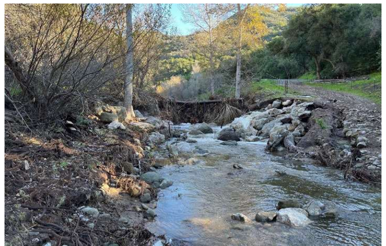
Figure 5-11. Modified Main Branch Maria Ygnacio Debris Basin w/ Rack Full of Debris, looking upstream (January 17 2023)
