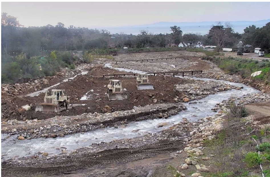
Figure 2-4. De-silting post-debris flow.
