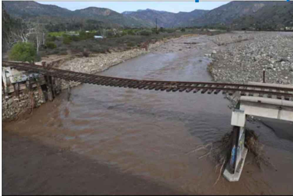
Missing Railroad Span Old Telegraph – Sespe Creek (VC Star)
