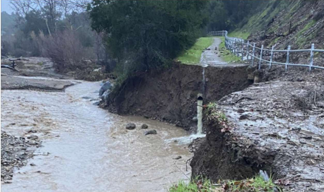
Ojai Valley Sanitation District broken pipe (Ojai Valley News photo)
