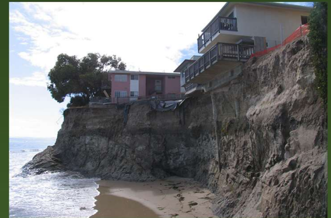
Eroding bluffs in Santa Barbara
